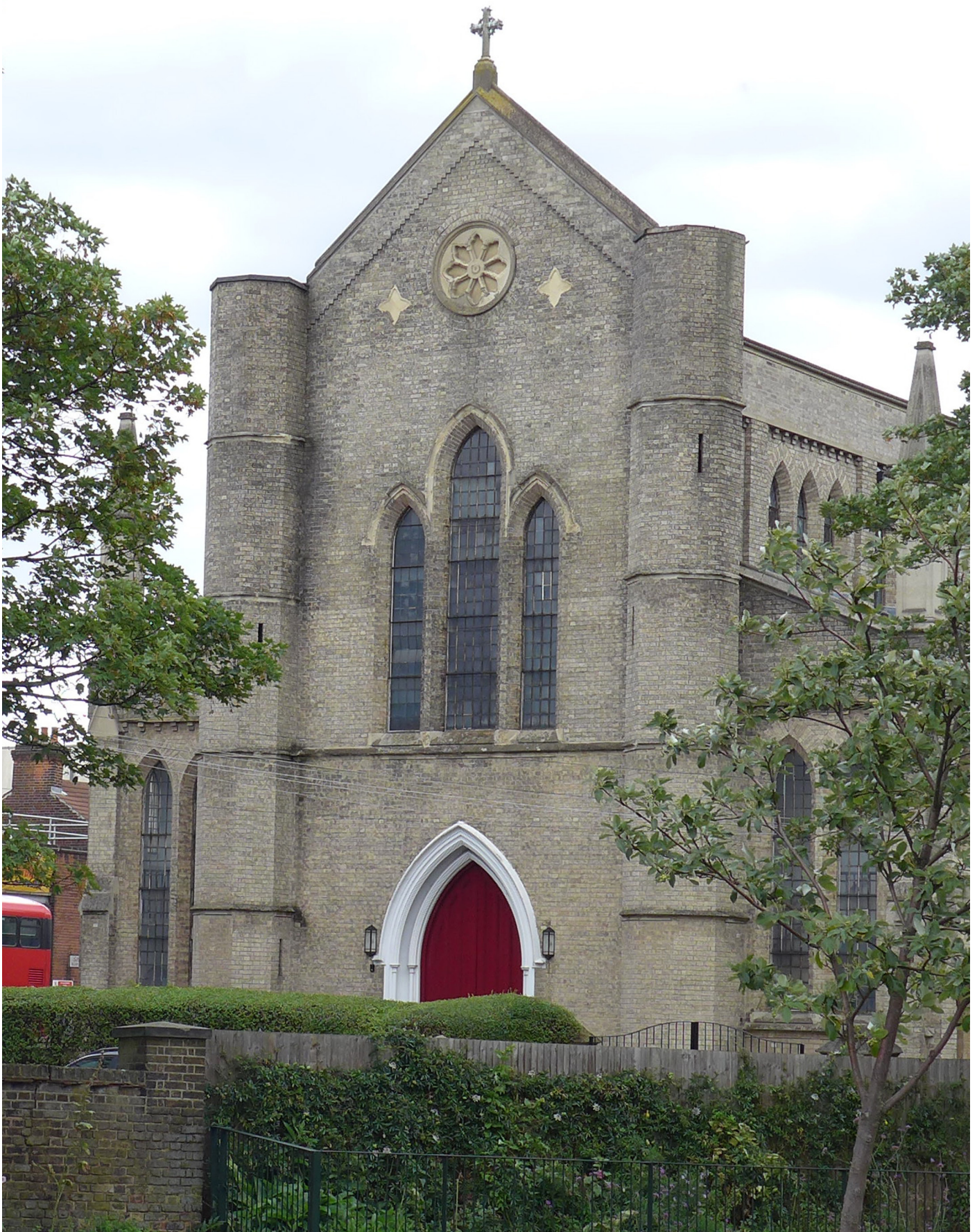
The west gable. The organ case abuts the badly damaged three lancet window in the west gable.
